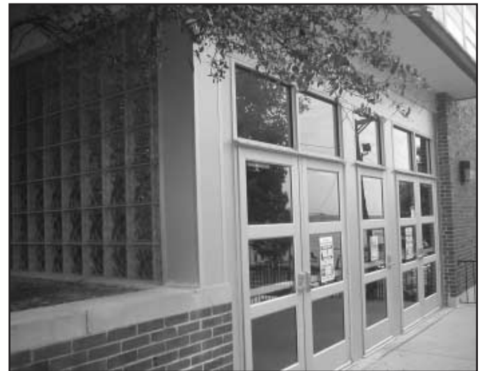
A new entrance was added to the gym area on Easton St. this summer.
